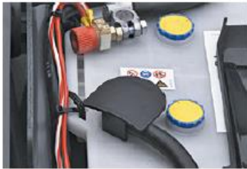
SmartCharge with fuse directly connected to the tractor's battery terminal.
