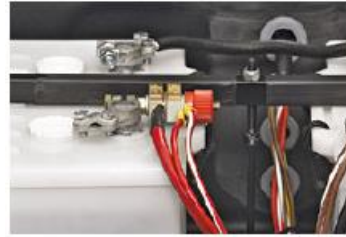
Battery connection at the trailer similar to the tractor. Feedback signal is realized by a crimp connection.
